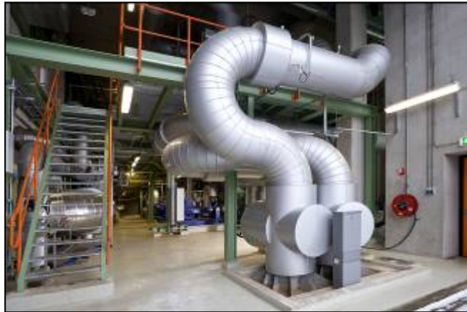
Warmtelevering Essent (80 MW)
